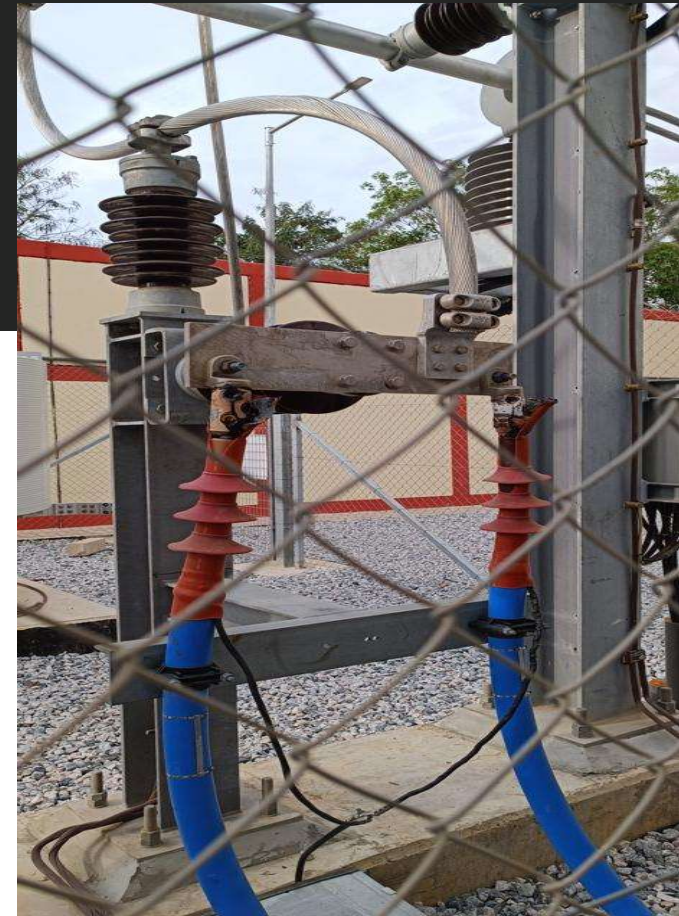
Kasoa Substation Damage to underground cables evacuating power from the substation
