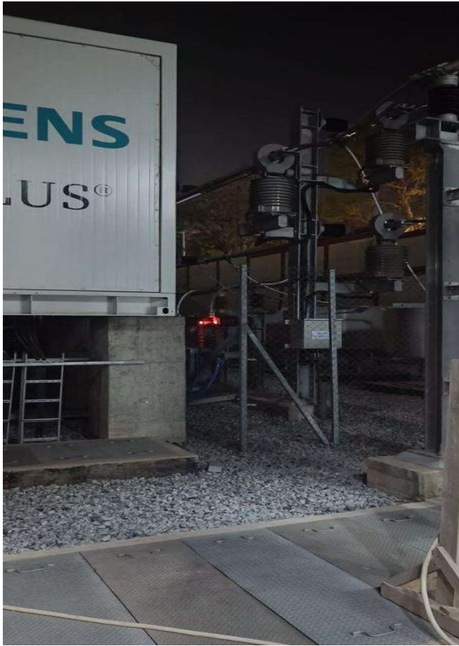
Kasoa Substation Hotspot on the Terminal (SVC)
