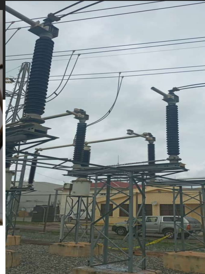
Aboadze Substaion: Damage to disconnect open and close terminal
