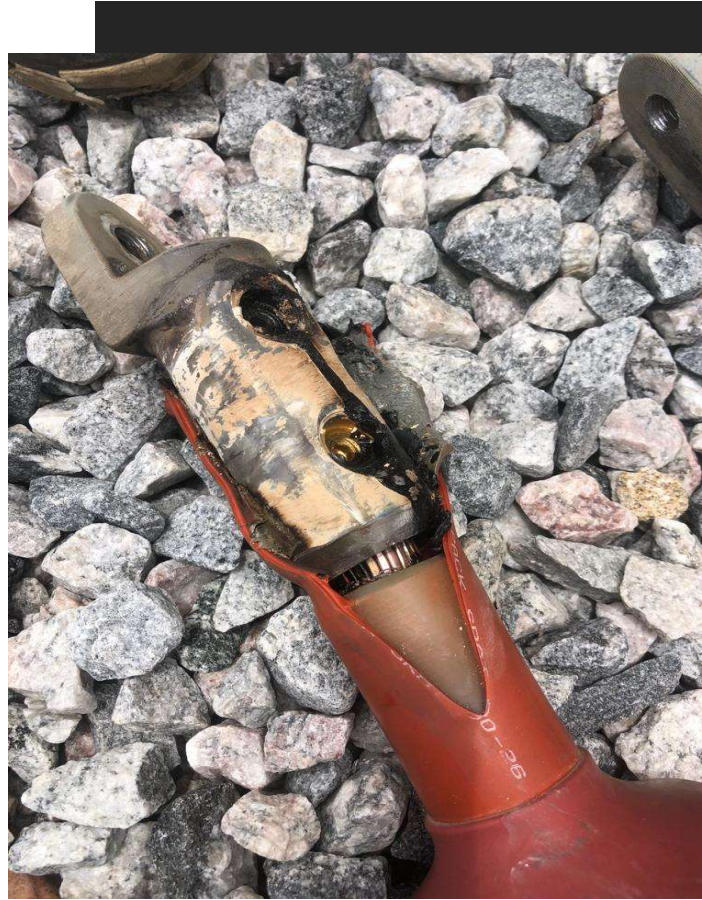
Kasoa Substation Damage to underground cables evacuating power from the substation
